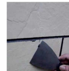
Remove excess adhesive or grout from the surface with a putty knife.
